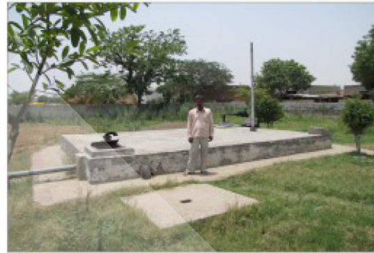
Figure 5. Sump of 50,000 ltrs with Booster pump of PHED, Haryana. Two tube-wells, each of 7.5 HP submersible pumps feed this sump. 35 year old one at 1 km delivers saline water, while 3 yr old pump at 2 km provides fresh drinkable water.
